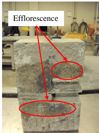
Figure 4.5. Efflorescence on specimen SP3-CI-10
